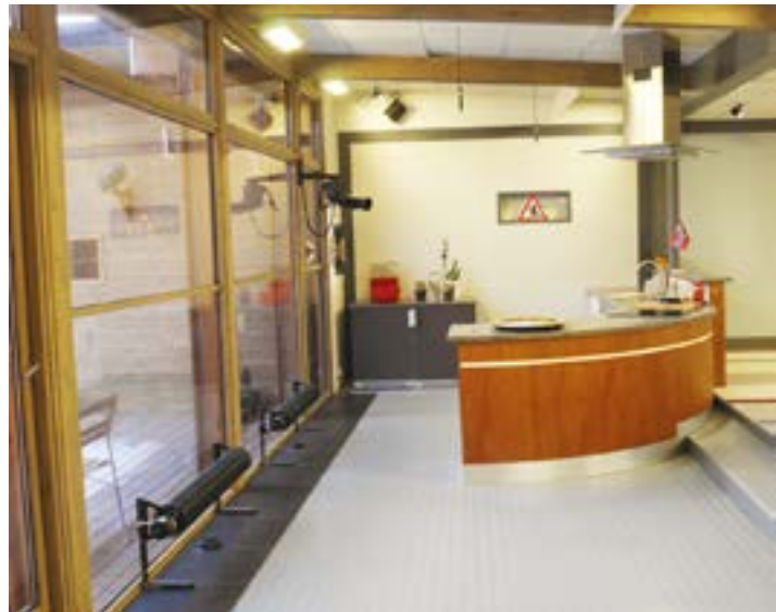
Installed by a window the ribbed pipe radiators effectively counteract cold draughts that frequently form by large glazed areas.
